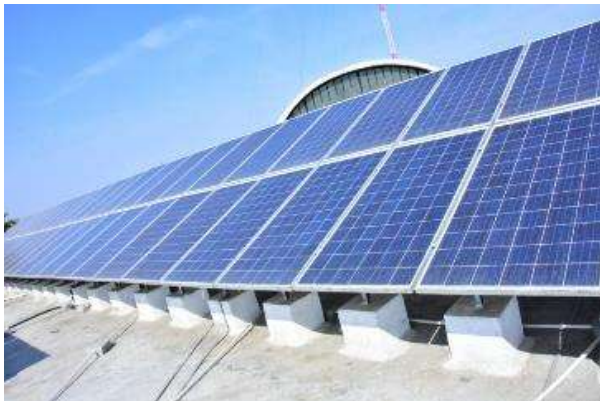
330 KW Solar Power Generation System & Solar Water heaters in all hostels
